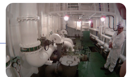
펌프설비 Cargo Pump Room
