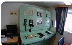
펌프실 Cargo Control room
